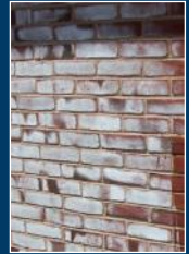
Efflorescence (calcium chloride)
